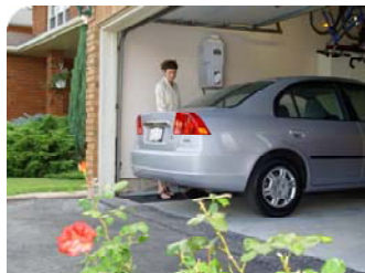
NGV Filling Station
