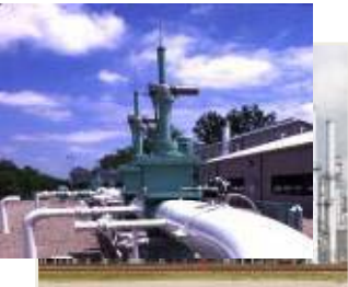
Pipeline / Chemical Plant
